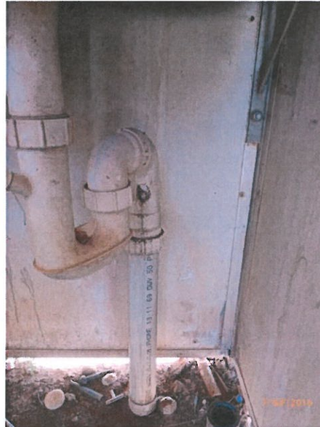
House 6 – Broken drain beneath bathroom sink – Repair.
