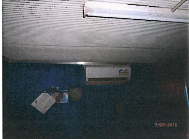
House 28 – Tenants complain that gaps in the wall junctions allow large amounts of dust to get into the room.
