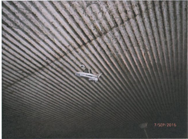
House 7 – Broken smoke alarm – Repair.
