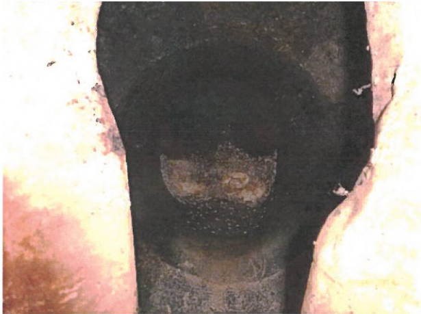
House 9 – Dry type septic tank full to capacity. Pump out.
