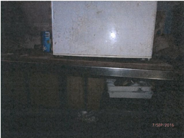
House 9 – Gap left when stove top removed repaired with unfinished plywood board. Inappropriate material for kitchen benchtops (refer to National Indigenous Housing Guide). Consider using an alternative robust material such as stainless steel or galvanised metal.
