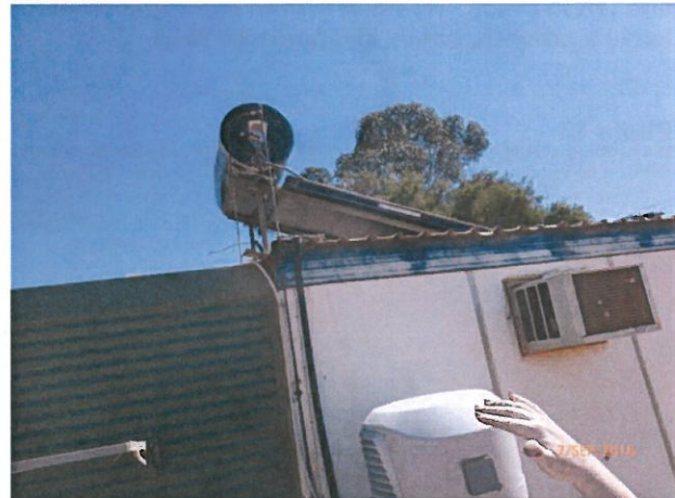
House 10 – Decommissioned and disused HWS is still connected to water and is leaking. Repair/remove HWS.
