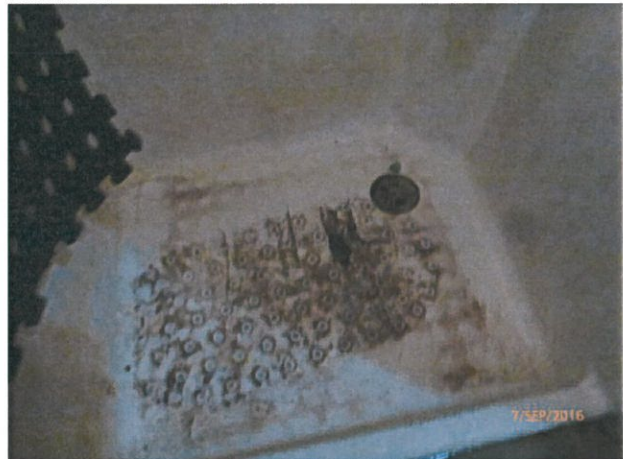
House 28 – Multiple splits in shower setting floor allowing water to penetrate into the structure of the bathroom, causing mould and deteriorating wooden floor and walls. Replace setting.
