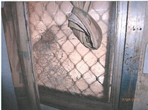
House 10 – Broken window in main transportable building. Repair.
