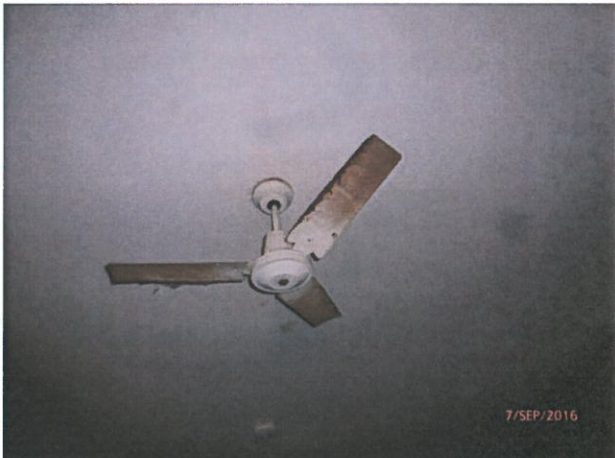
House 9 – Bent ceiling fan in lounge room. Repair.
