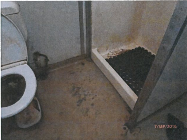
House 28 – Mould in flooring caused by water penetration from shower setting.
