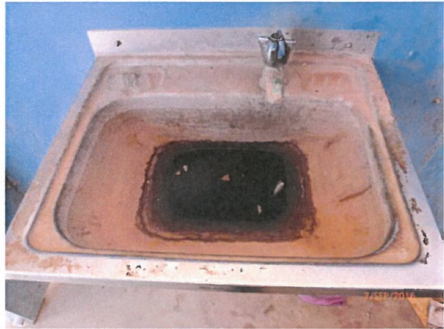
House 1 – Blocked Sink
