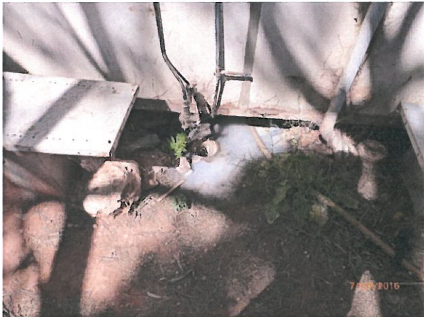
House 28 – Plumbing from bathroom apparently broken with waste water flowing onto the ground beneath house without treatment. Repair pipes to compliantly direct waste water to a working sewage treatment system.
