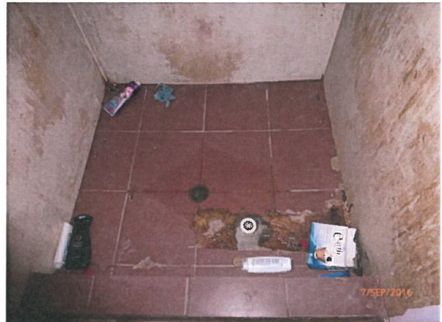
House 5 – Ad hoc repair of shower gully leaving surface unfinished and water pooling in old gully. Unsanitary and non-compliant construction. Please repair to leave a surface that is impervious to water and graded to the gully such that no pool is able to pool.
