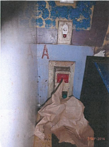
House 9 - Disconnected hot plate switch broken and left in place. Remove switch and repair wall to leave a smooth, easily cleanable surface.
