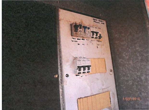
House 5 – Fuse appears to be tripping, affecting power to fans and power plugs along the southern side of the dwelling.
