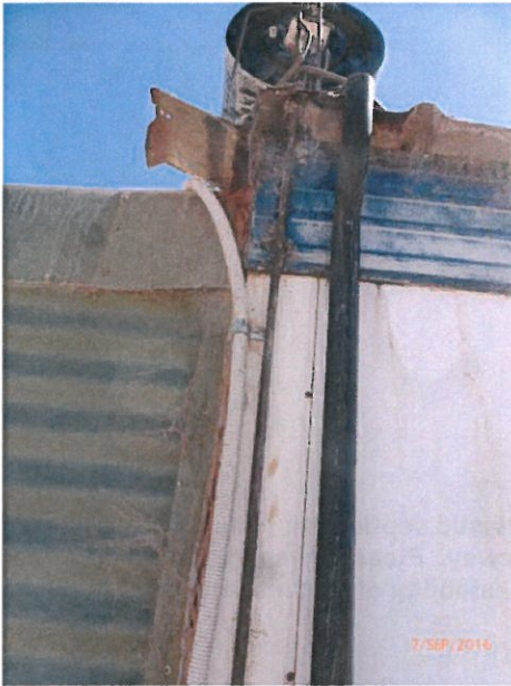
House 10 – Water leaking from HWS flowing down water pipes.
