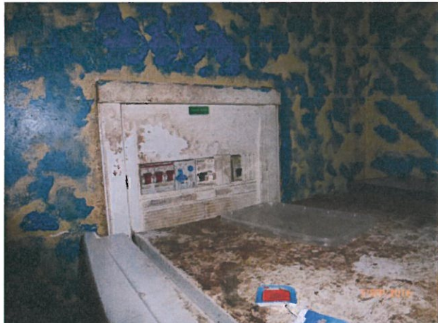
House 9 – RCD is continually tripping. Electrical fault. Repair.
