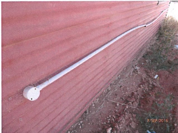
House 5 – Electrical installation ducted approximately 1 metre above ground. This is believed to be a safety hazard and non-compliant with electrical safety standards. Please rectify.
