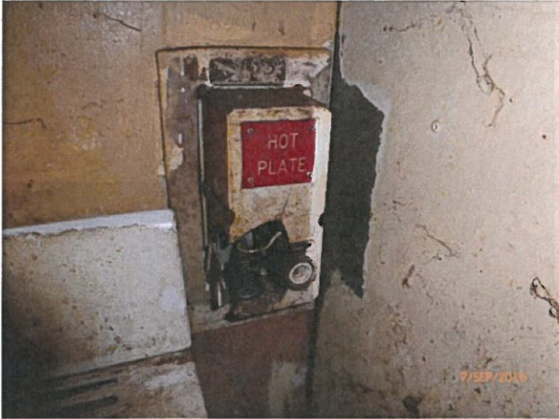
House 6 – Disconnected hot plate switch broken and left in place. Remove switch and repair wall to leave a smooth, easily cleanable surface.
