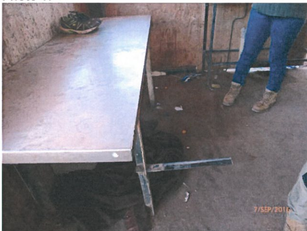
House 6 – Damaged bench seat leaving protruding joists. Dangerous condition presenting a trip/fall hazard to the tenants. Repair.
