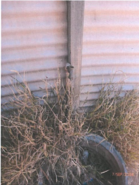
House 6 – Broken toilet tap – Repair.
