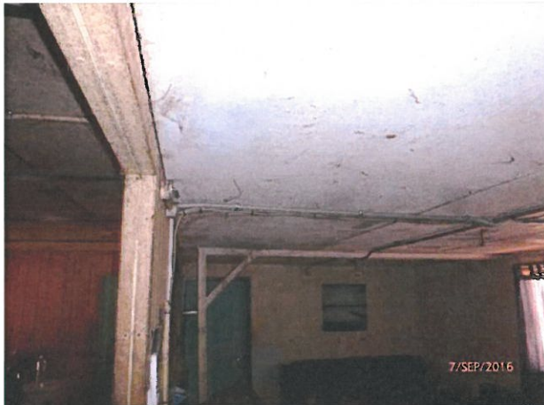
House 10 – Extension from main transportable. Please review the method of joining the buildings together as the extension is subsiding with floor and ceiling now set on an angle slanting away from the main transportable.
