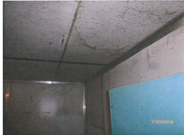
House 10 – Water is leaking into the room from a leak in the decommissioned hot water system (HWS) on the roof. Adequately remove water supply from disused HWS.
