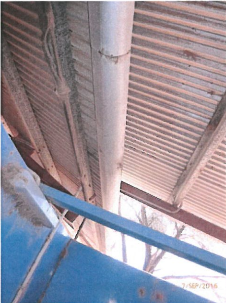
House 9 – Blocked gutter causing collected water to leak in shower. Unblock built up leaves etc. from gutter.
