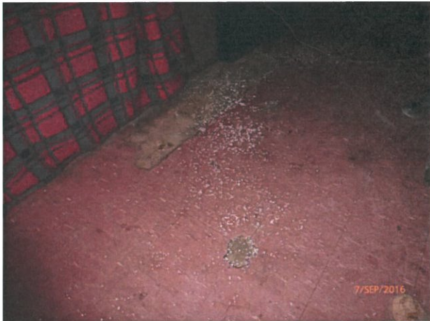
House 7 – Wall insulation on floor indicates presence of rodent pests.
