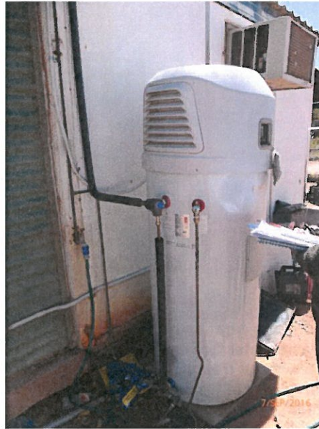
House 10 – New HWS installed but tenants report that they were not given instructions on how to operate the system and complain that they are receiving only lukewarm water.
