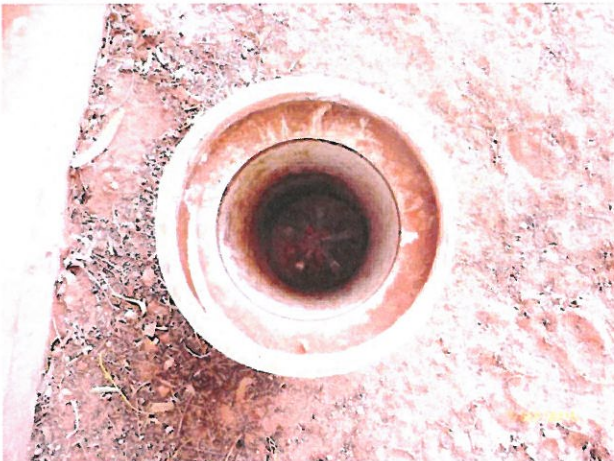
House 9 – Missing cover for disconnecter gully allowing items to be placed down pipe, like the bottle in the photo. Replace cover.
