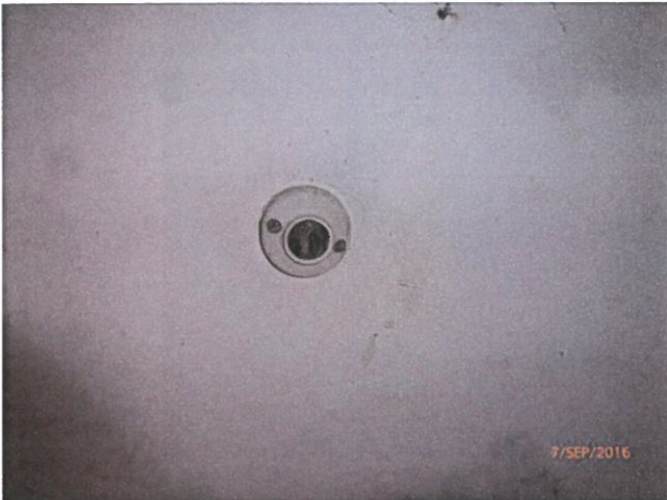
House 5 – Damaged light fitting in bathroom where fitting has been removed leaving bathroom without adequate lighting. Repair/replace fitting.
