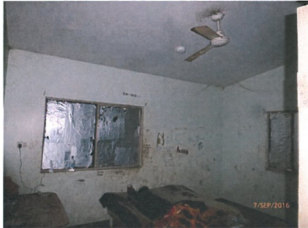
House 9 – No electricity to bedroom and broken ceiling fan. Repair electricity supply and fan.
