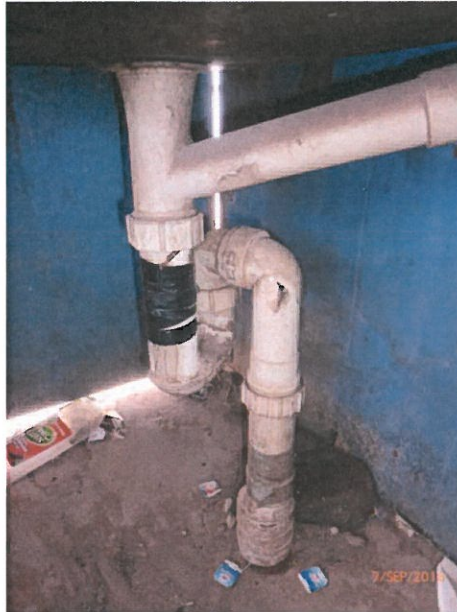
House 1 – Broken waste pipes from laundry basin. Non-compliant drainage. Replace broken plumbing.
