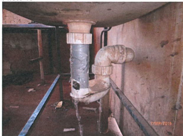
House 6 – Broken drain beneath external veranda sink – Repair.
