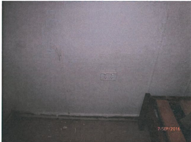
House 5 - Fuse appears to be tripping, affecting power to fans and power plugs along the southern side of the dwelling.
