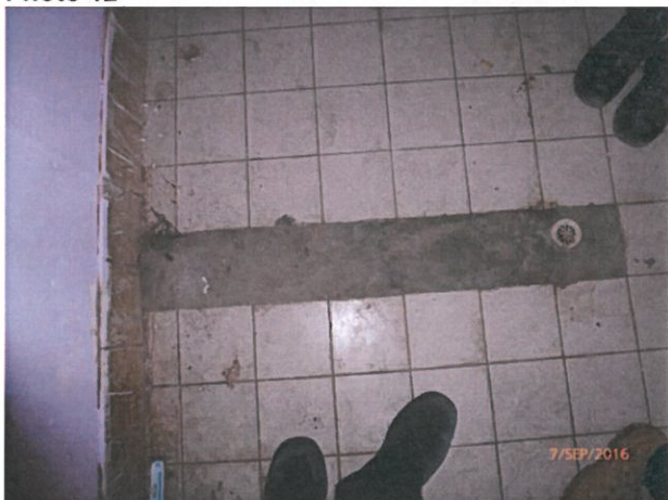
House 5 – Ad hoc repair on bathroom floor leaving surface unfinished. Please Repair.
